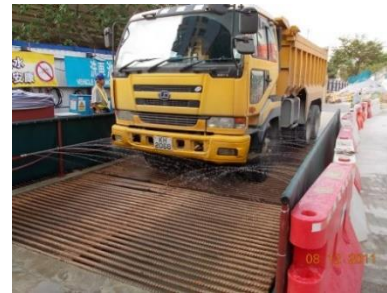
Wheel Washing Facility
